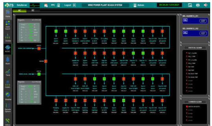
Figure 19. Auxiliary Power Supply Monitoring
