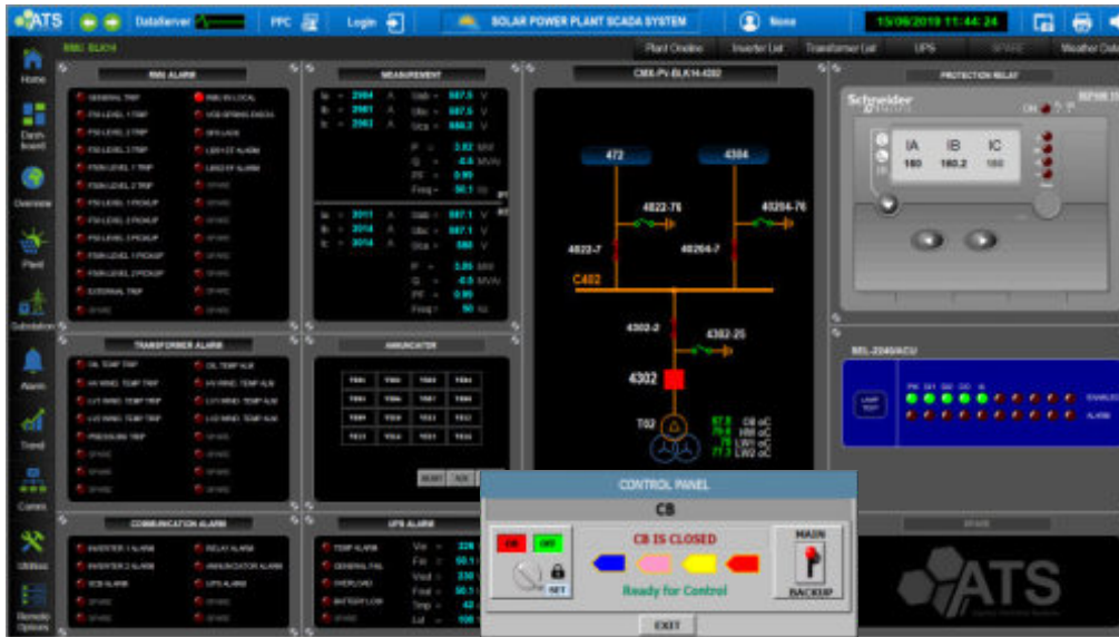
Figure 8. RMU Breaker Control
