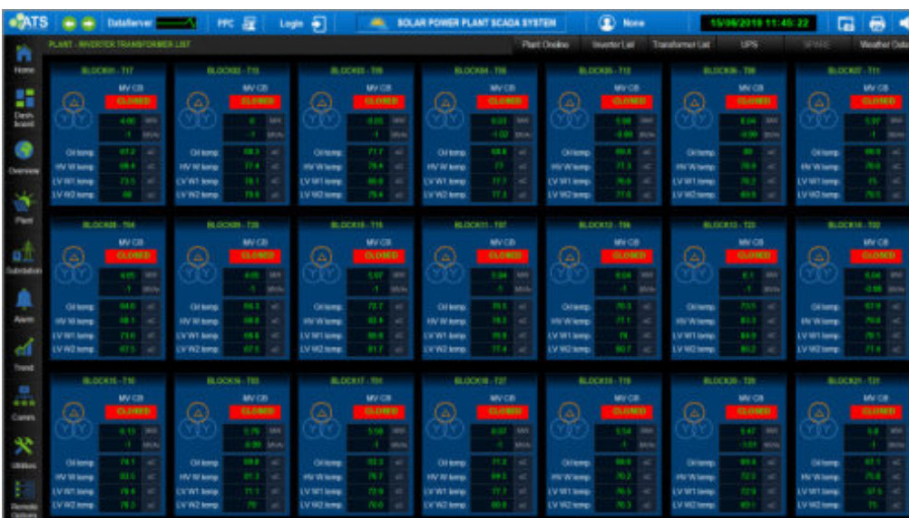
Figure 13. MV Transformer Monitoring
